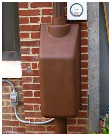
Figure 7. Low-pressure vacuum gauge and sensor.
