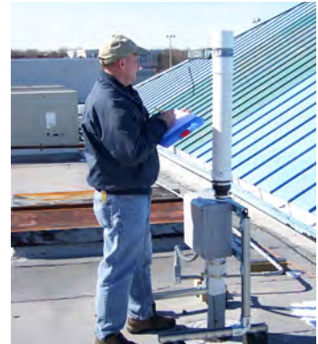
Figure 9. Blower exhaust airflow performance testing for total system.
