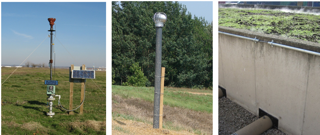
Figure 1. Examples of passive control options for sustainable gas management: solar spark “tiki-torch” (left), “whirlybird” vent (center), or biofilter (right) (Courtesy of Geosyntec)
