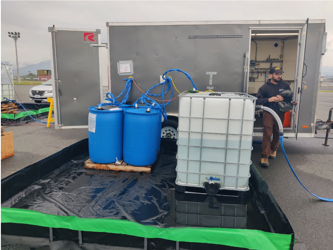
Trailer, F400 GAC drums and effluent tank (Kornuc 2024)
