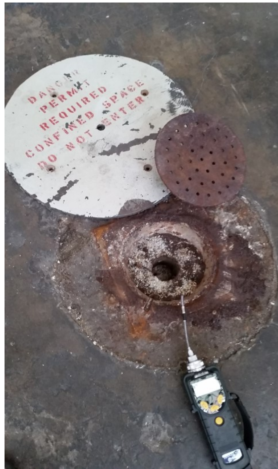
Figure 2. Vapor Intrusion entry point and a PID.
