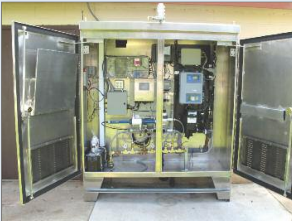
Water quality monitoring equipment panel installed at the Pleasant Valley site, Naval Base Ventura County.
