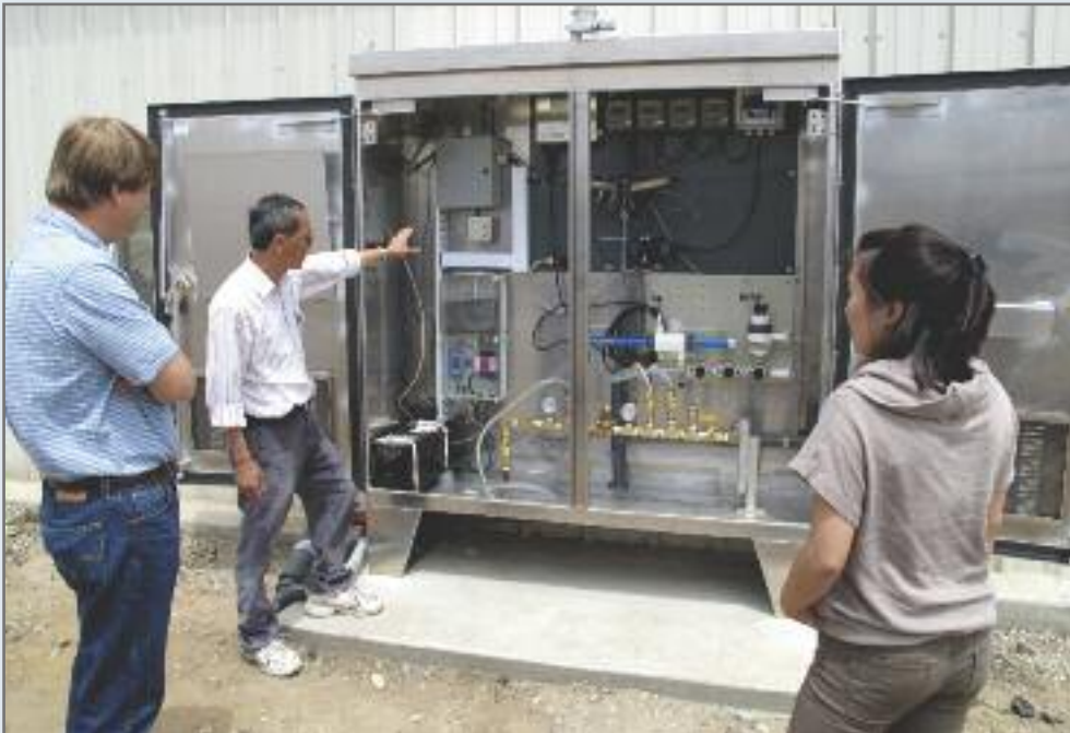
(from left) Ken Kaempffe, Steve Fann, and intern Lauren Kim inspect the water quality monitoring equipment at the Pleasant Valley site, Naval Base Ventura County.
