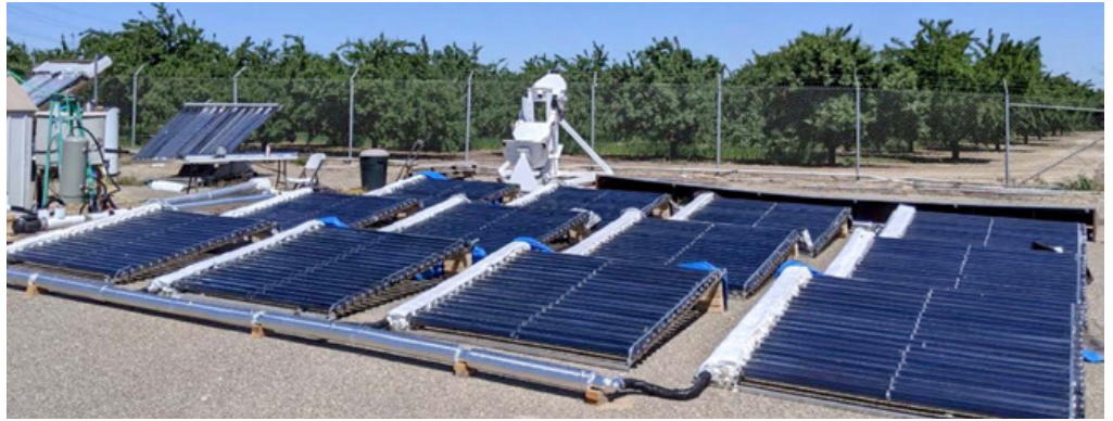
The XCPC system. (Photo Credit: Winston Cone Optics)
