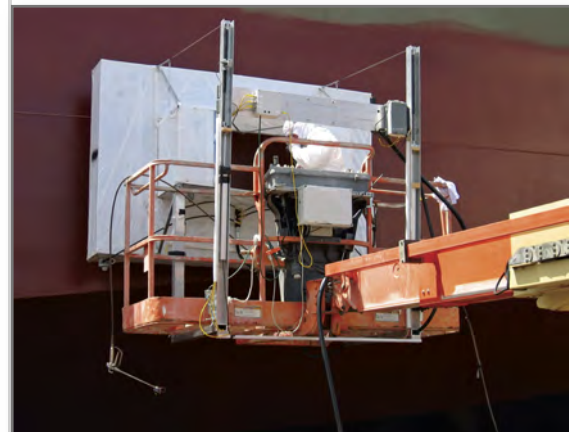
The MAEE can be assembled on a conventional boom lift in approximately one hour.
