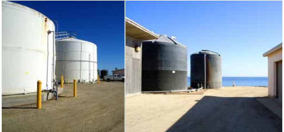
Navy drinking water treatment facility with potable treated water storage tanks and reverse osmosis tanks. (Photo Credit: Autumn Resto)
