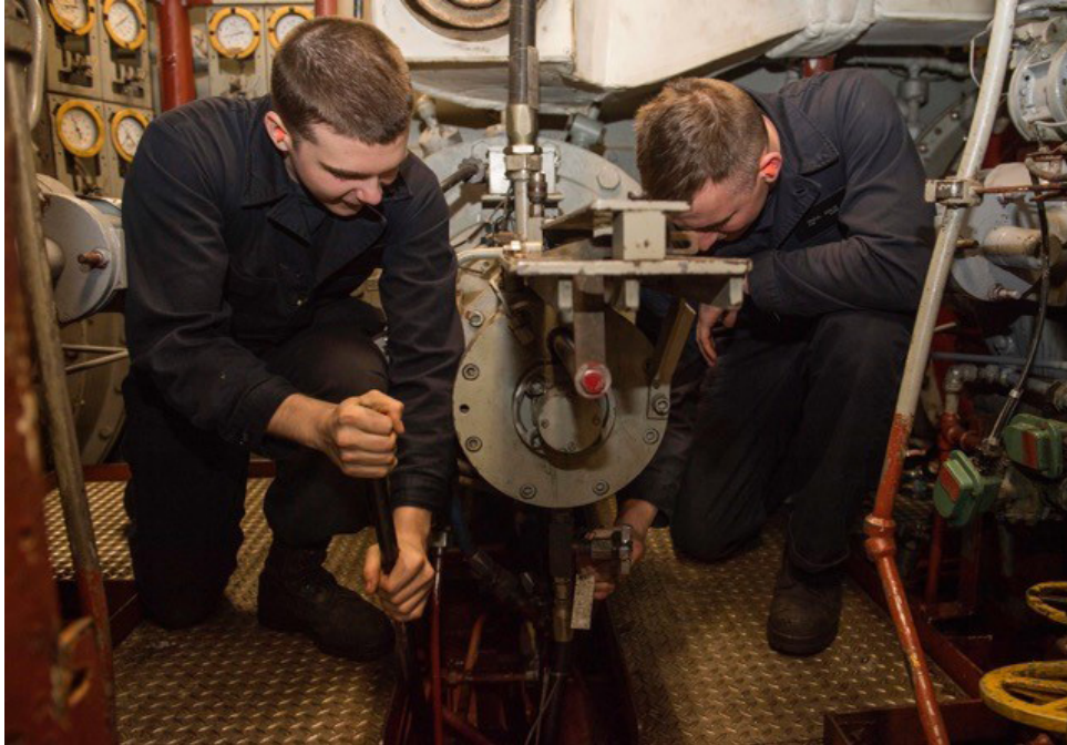
Two firemen clean the bilge aboard USS Oak Hill (LSD 51). Bilge water impacted by PFAS is one of the potential waste streams that this project is addressing. (U.S. Navy photo by Mass Communication Specialist 3rd Class Jessica L. Dowell)
