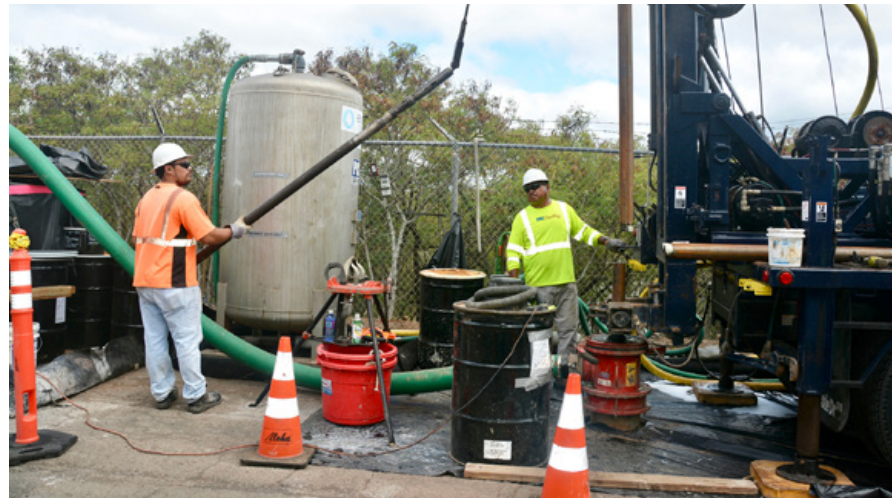
Soil and/or wastewater from well installations can be a source of per and polyfluoroalkyl substances. (Photo Credit: Theanne Tangen)
