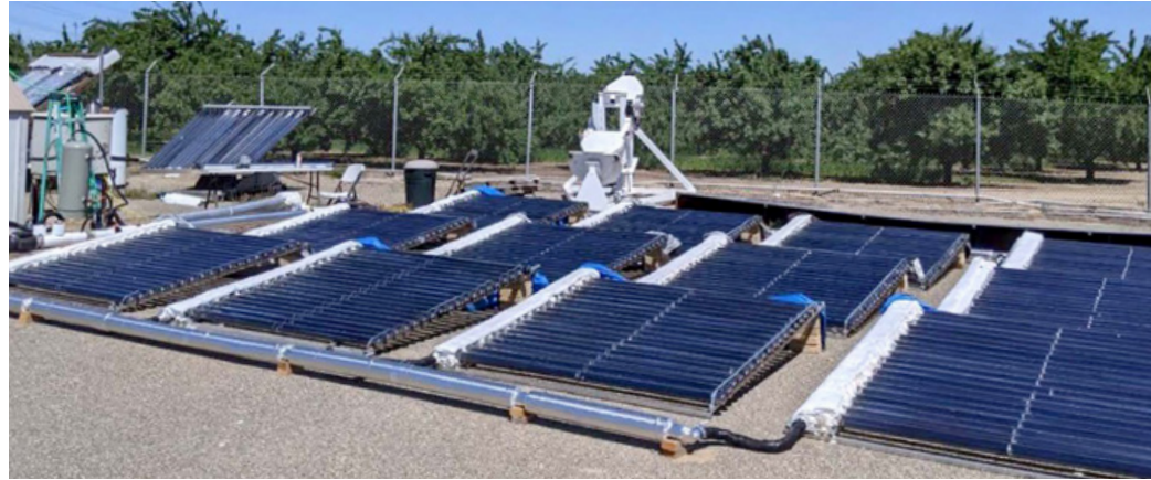
The XCPC system. (Photo Credit: Winston Cone Optics)
