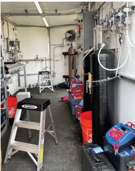
Pilot treatment trailer containing sorption units and sonolysis reactor to be used for this project's field effort.
