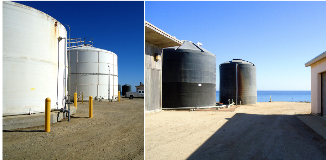
Navy drinking water treatment facility with potable treated water storage tanks and reverse osmosis tanks. (Photo Credit: Autumn Resto)
