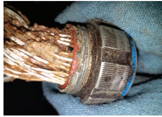
Degraded wires from the V-22 Osprey Full Authority Digital Engine Control (FADEC) and Flight Control Wiring.
