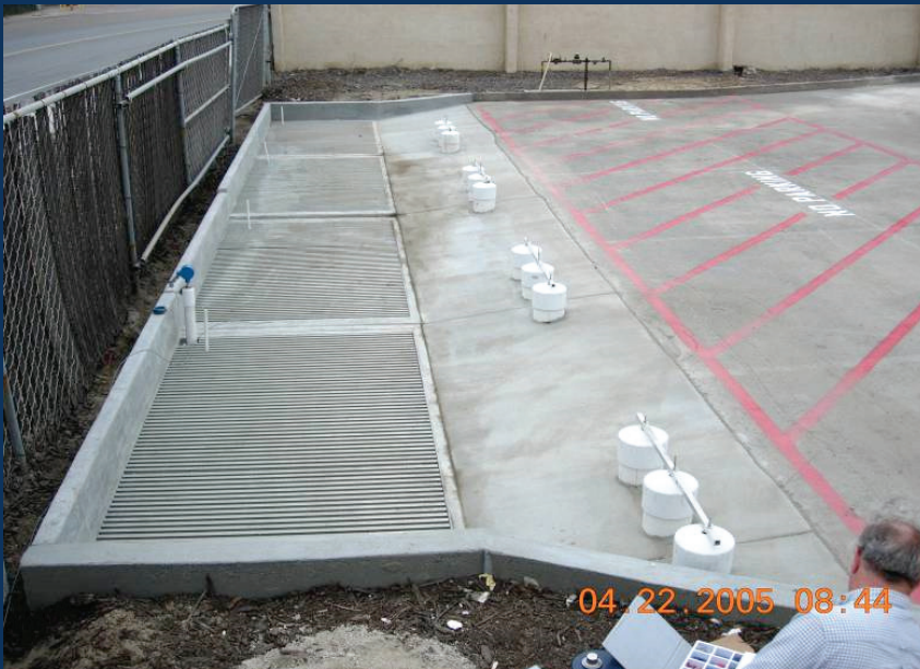
Installation of Structural BMP at Naval Base San Diego Recycling Center – NESDI Project 454. (Photo credit: Gary Anguiano)
