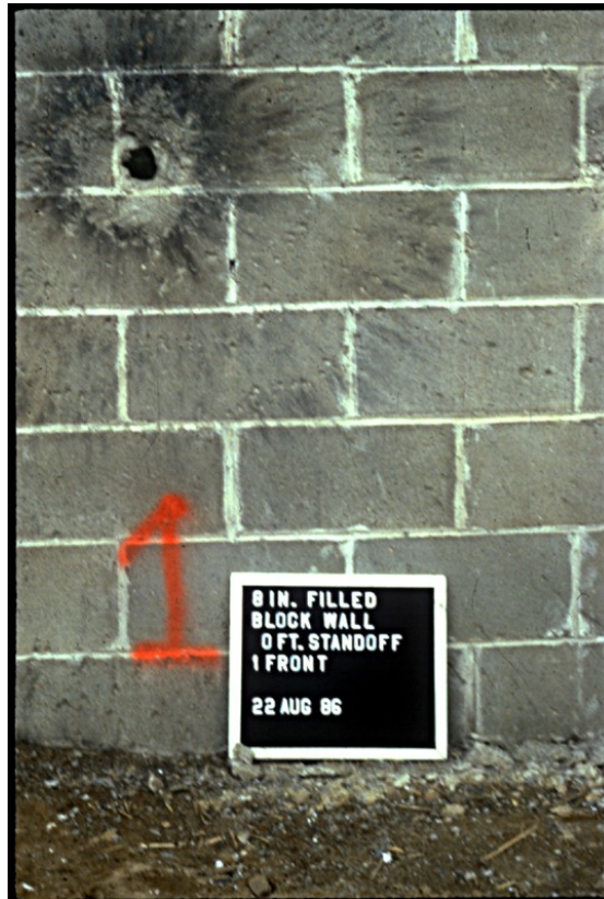
Figure 2-3. Shaped Charge Penetration of Masonry
