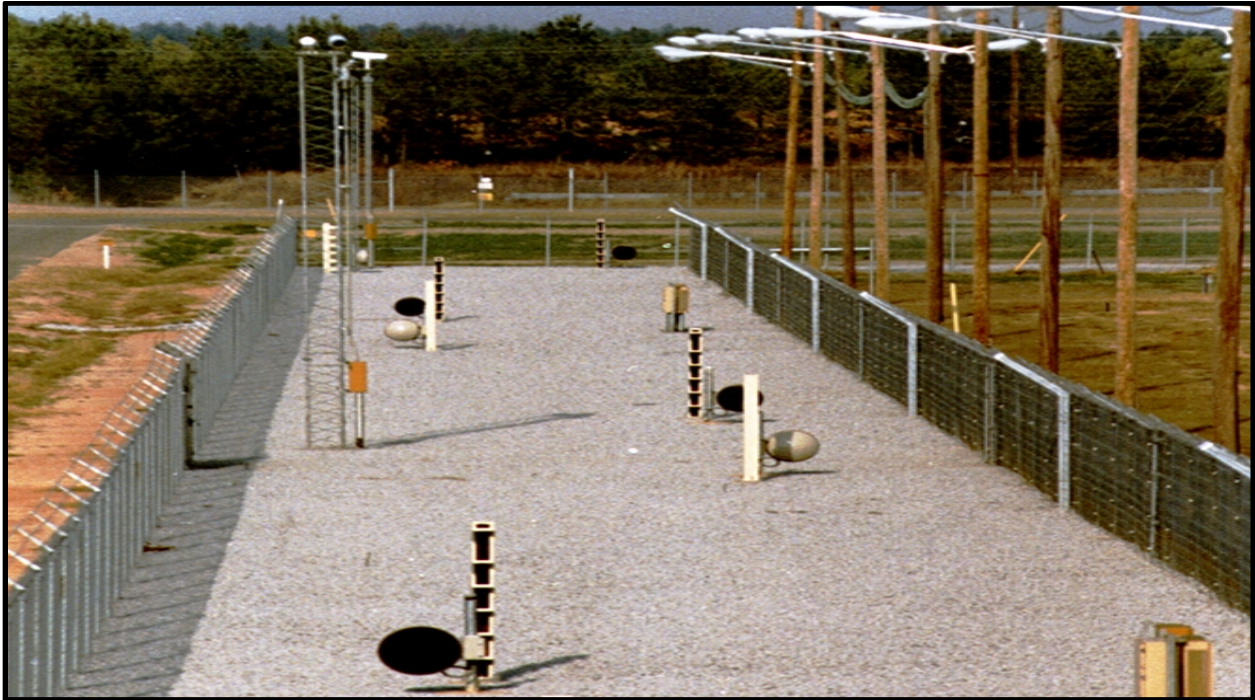
Figure 2-7b: Double Fence Line
