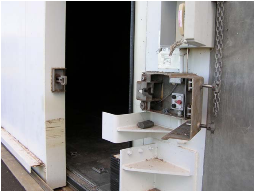
Existing Door with 833 Padlock and Universal Security System
